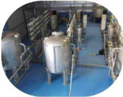
Reverse Osmosis Desalination
